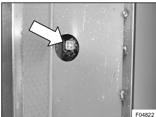
Figure 29: Socket at LHS of main junction box (at RHS on multiplexed vehicles)
