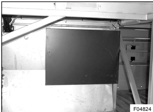
Figure 3: HVAC junction box (in the luggage compartment)
