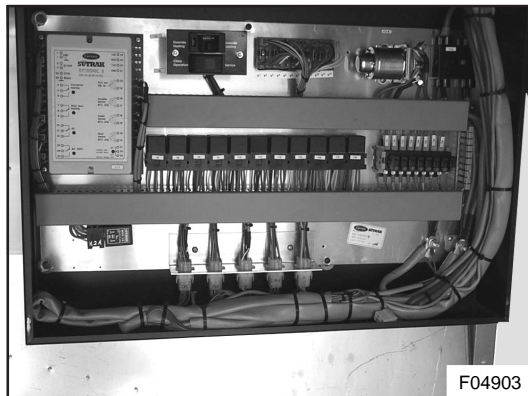
Figure 1: HVAC junction box in luggage compartment
